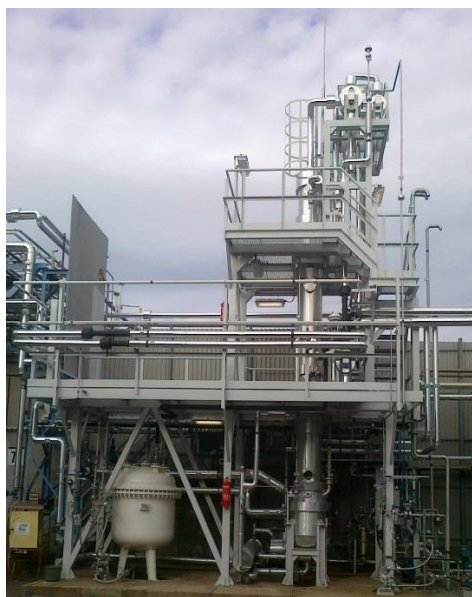
Figure 2, AOX removal column at EGIS Pharmaceutical
